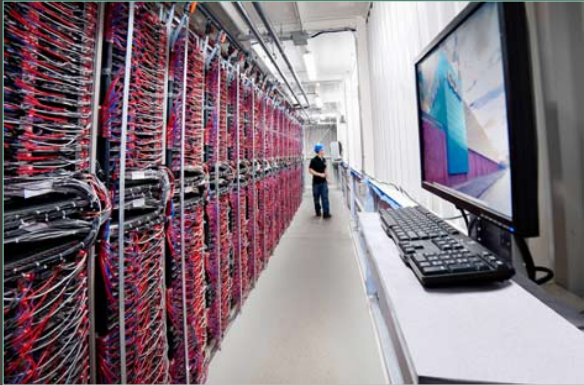
OVH server room ©OVH
